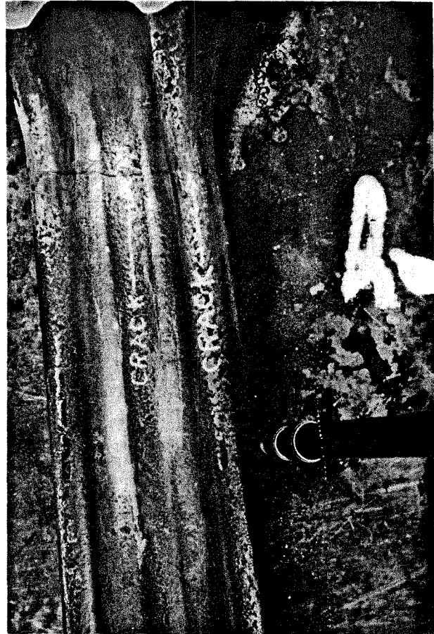
Figure 6. Close-up of another crack in a connecting rod. The crack was found during periodic inspection.
